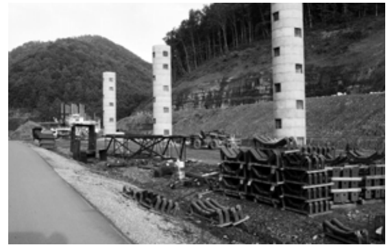
Fresh construction of a coal belt line is happening at the breach site of the 1972 Buffalo Creek coal sludge disaster.
