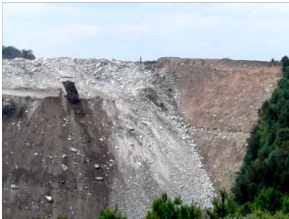
A little more of West Virginia's heritage goes tumbling out the back of a massive dump truck (upper left) at a valley fill in southern WV. The U.S. Army Corps of Engineers considers this type of destruction "minimal."
